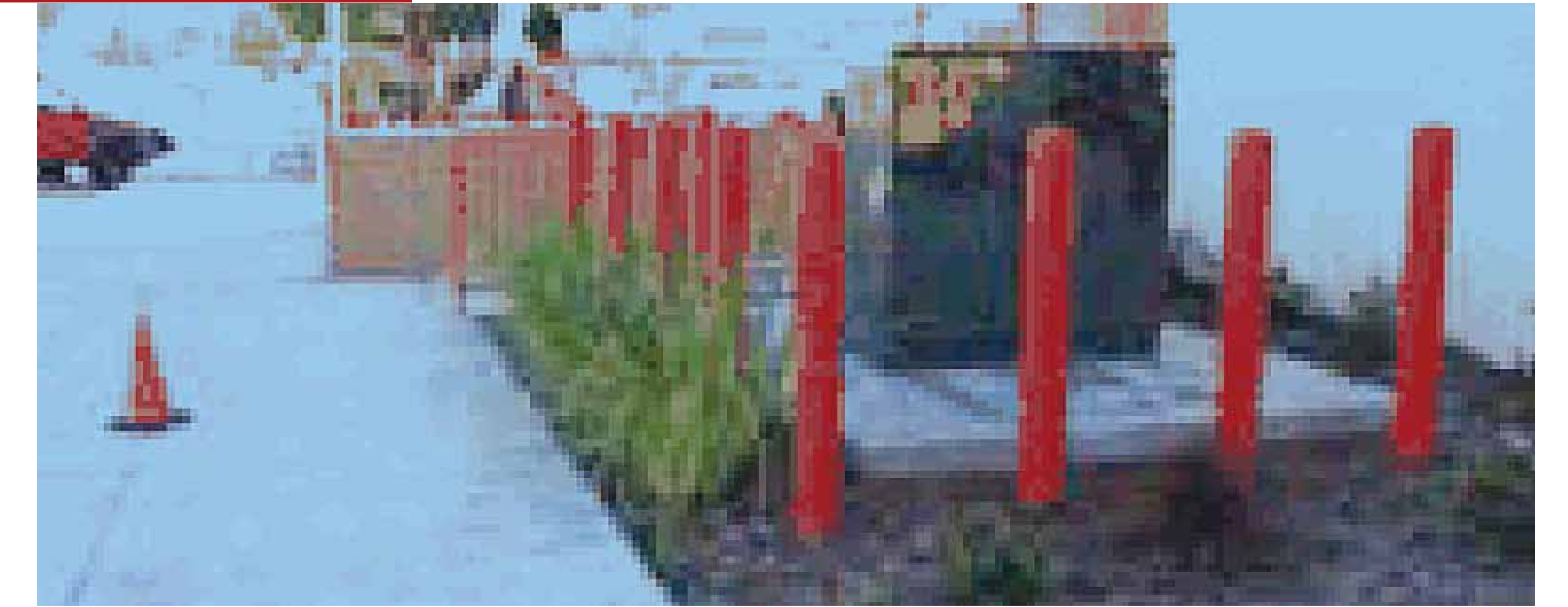
An example of poor equipment location choice. A primary opening to a courtyard garden is walled off with electric meters. The area could be better screened using landscaping.
